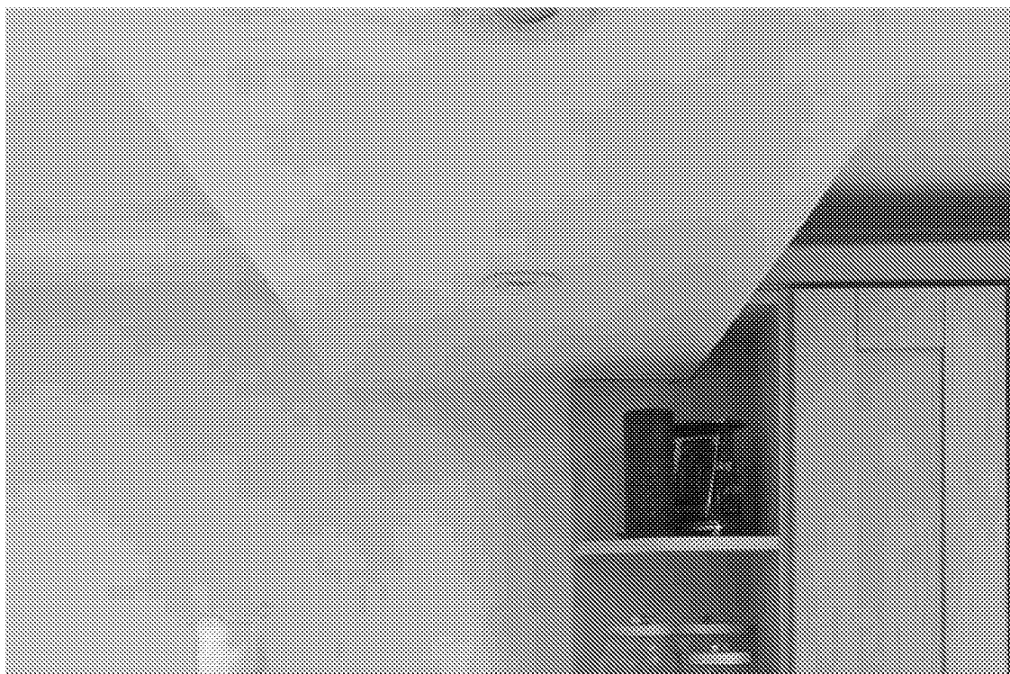
Fig 5: A full width beam has been inserted in the kitchen space where the chimney stack used to sit. Whilst the loss of historic fabric cannot be condoned, anything that replaces it can only ever be a replica and the existing beam does provide a profile in the living space, to allow for the appreciation of the former divide to be still clearly understood.
