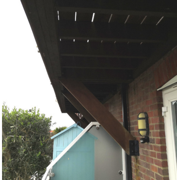
Supports to 32 and 33 Balconies
