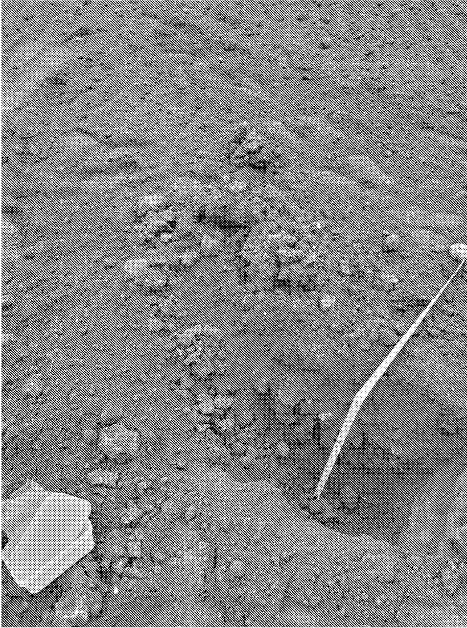
Photo of hole with tape in place
