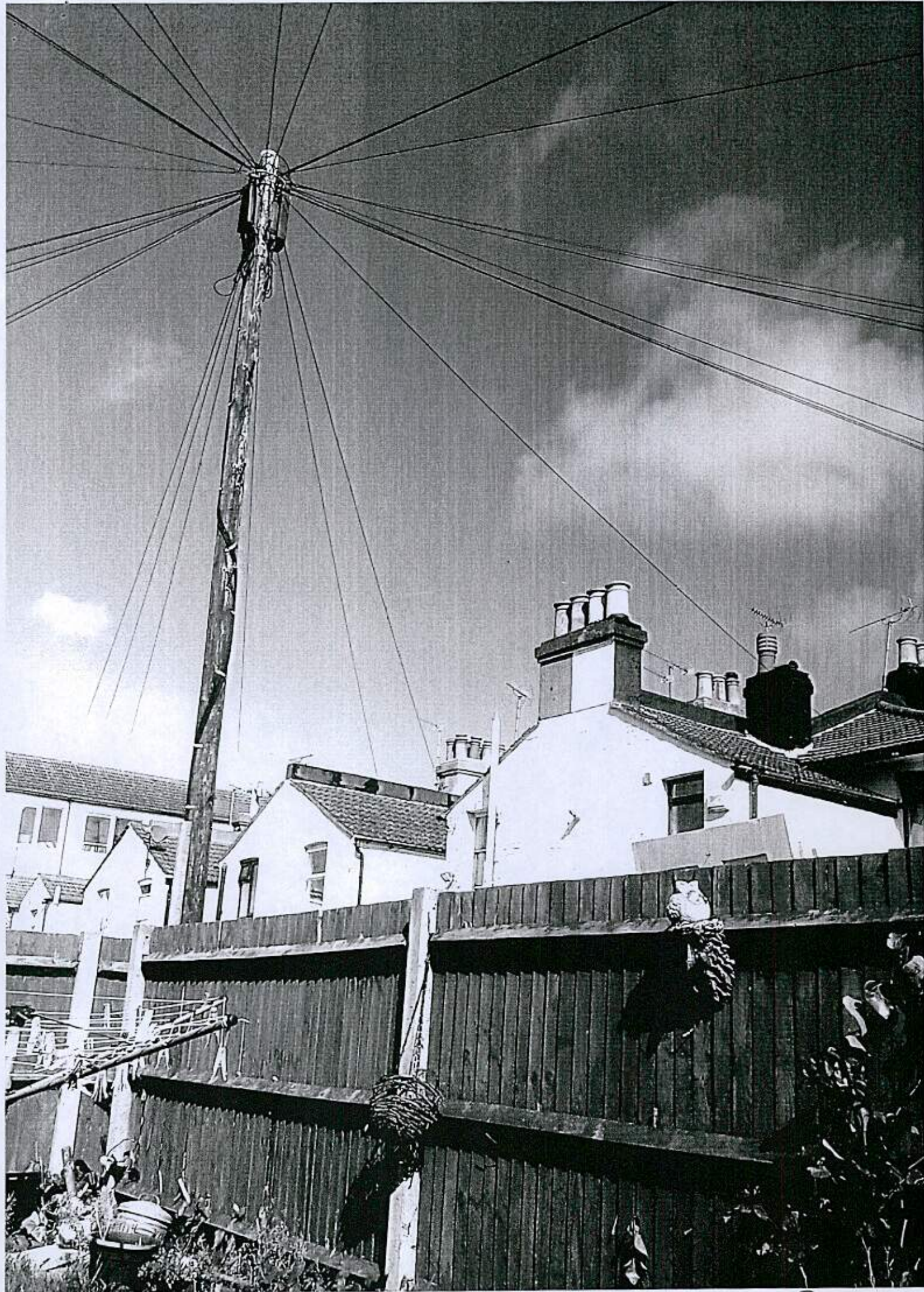
TELEPHONE POLE AT REAR OF 41 NEW ROAD
