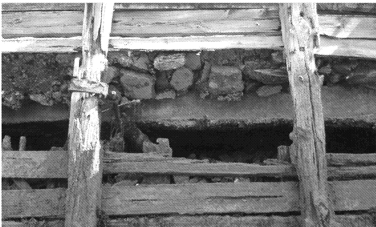
Photograph 2. Eroded cavity within existing flood defence wall. Note likely unsuitability of eroded cavity for nesting birds within breeding bird season (March – September) as indicated by presence of marine algae as evidence of regular inundation.
