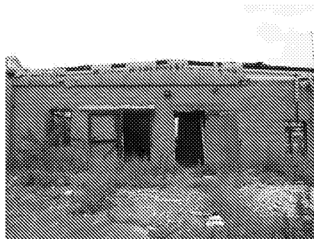
Photo 2. Fire damaged buildings
