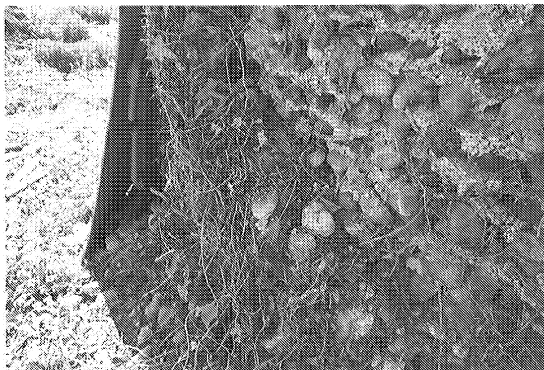
Photograph 6 – Loose flintwork adjacent door
