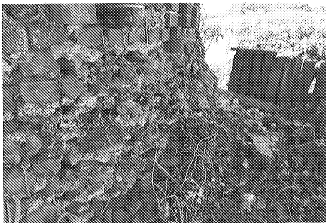
Photograph 8 – Collapse of flint skin
