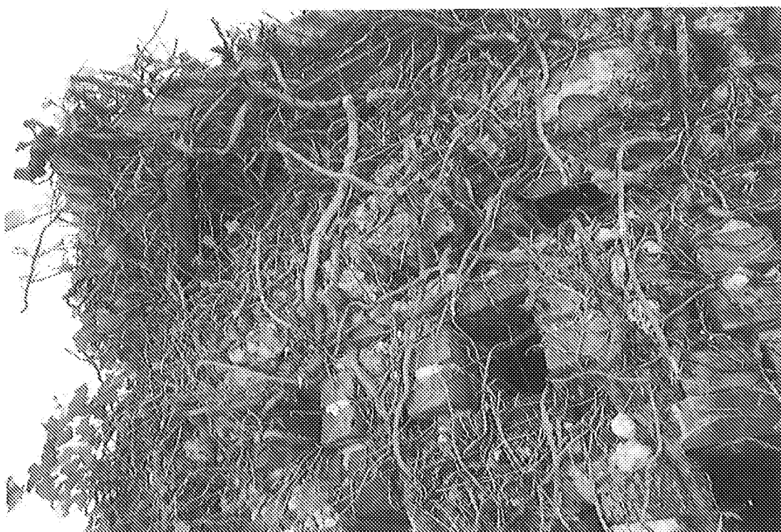
Photograph 7 – Extensive ivy incursions and flint skin collapsed
