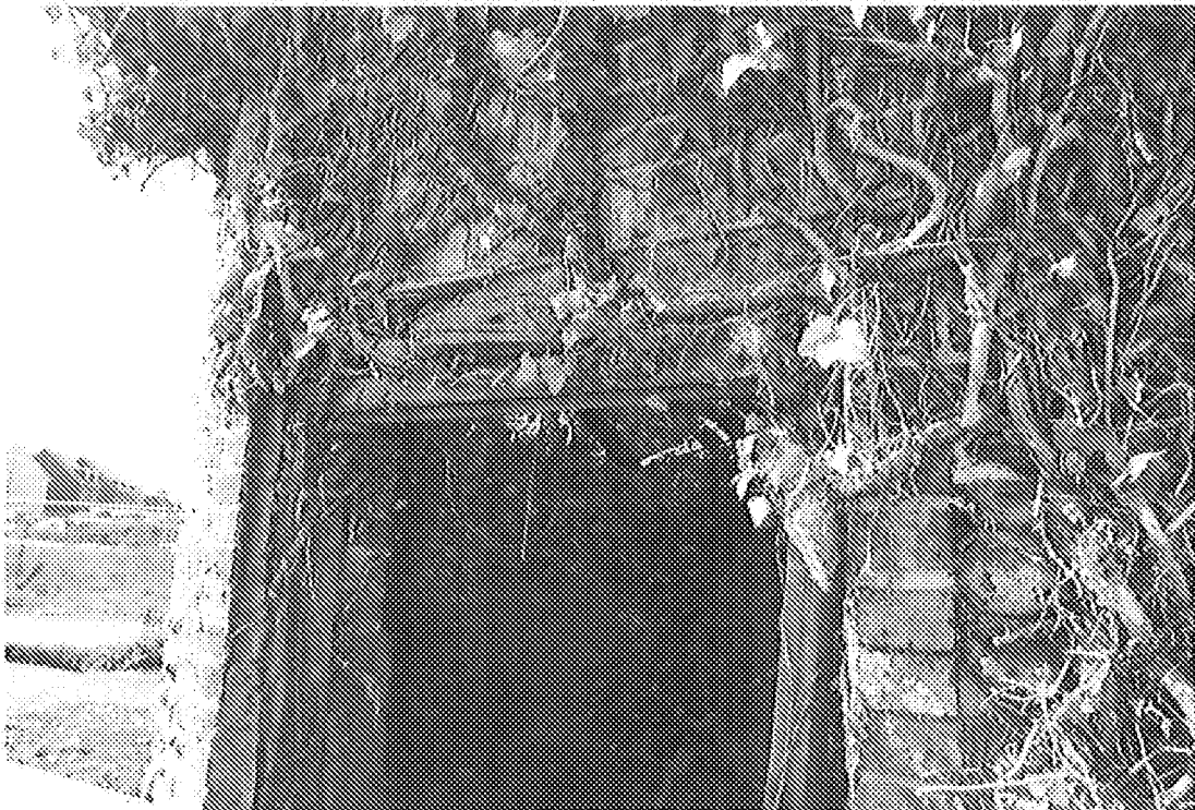
Photograph 3 – Ivy growth at entrance – timber lintel decayed
