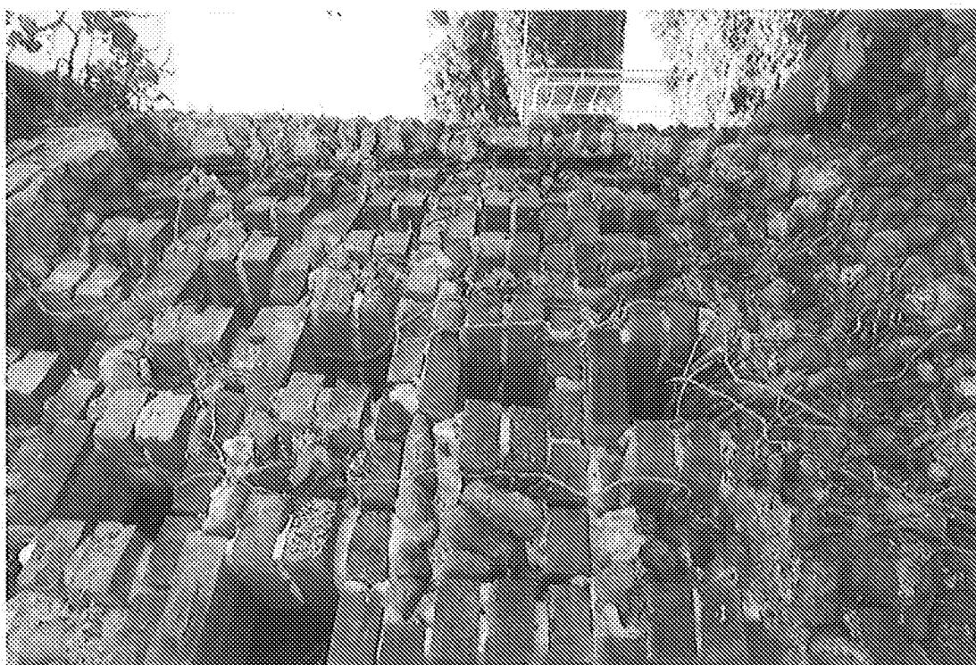
Photograph 9 – Collapse of flint skin
