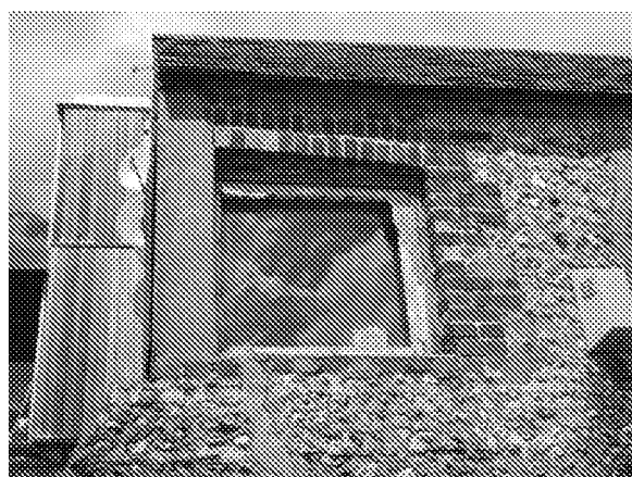
Figure 10: Truncated first floor window
