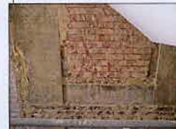
PHOTOGRAPH B BRICKED UP WINDOW OPENING AND RENDER SURROUND
