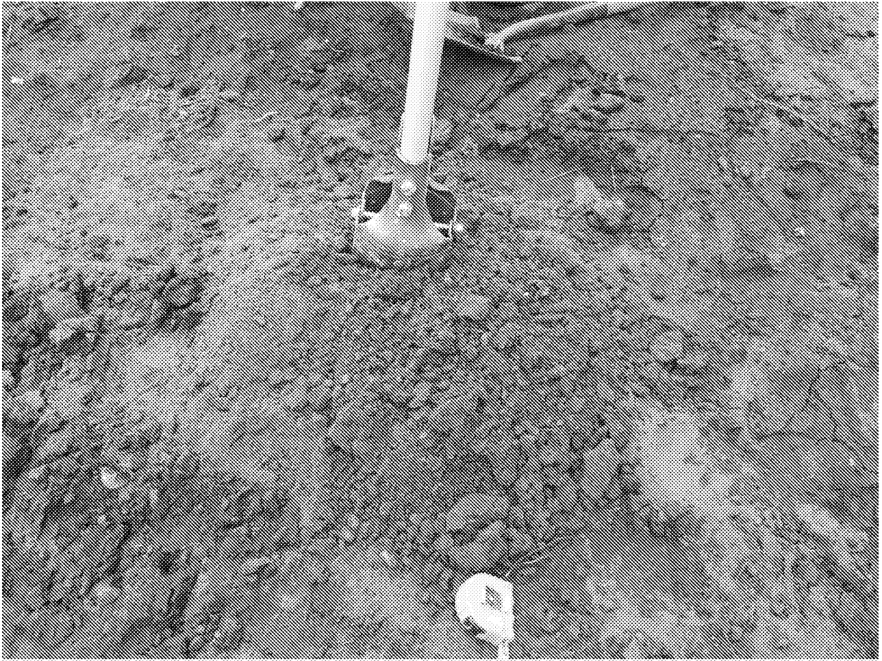
Photo of hole with tape in place
