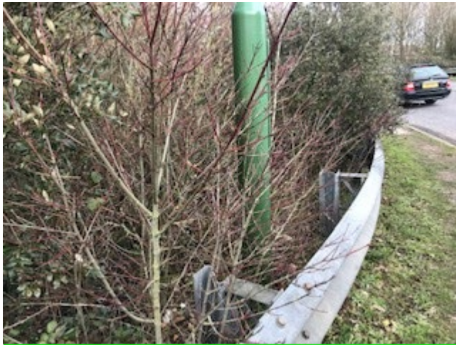
Figure 6: lamp column in the working width of the VRS.
