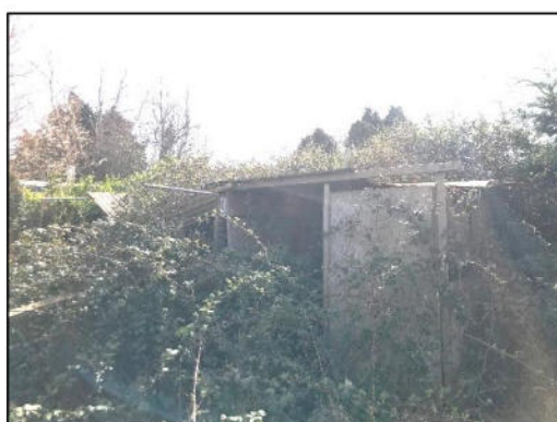
Figure 11: Dilapidated wooden shed overgrown with bramble
