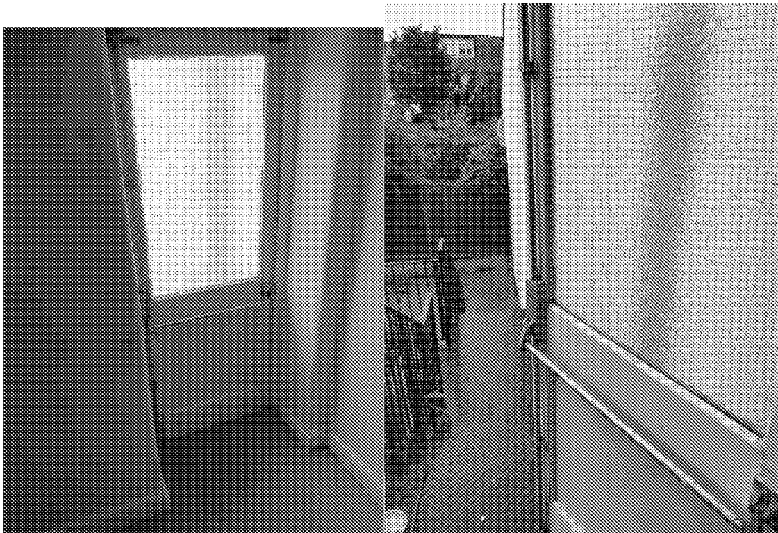
Photo 1 & 2: Existing fire door which exits to garden area.
