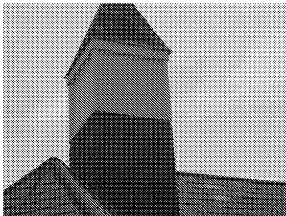
Clock tower, western aspect, missing/slipped hanging tiles
