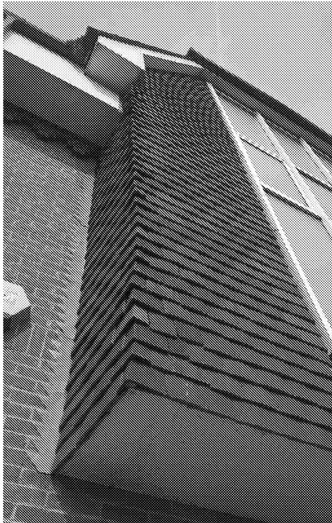
Plate 7 - Gaps present beneath the clay hanging tiles on the eastern side of B1.
