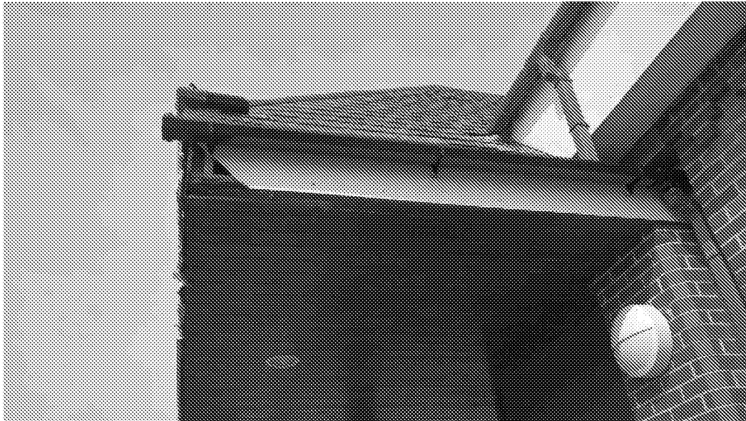
Plate 8 - Missing section of fascia board providing a potential access point into the soffit box at the south-west corner of the building.
