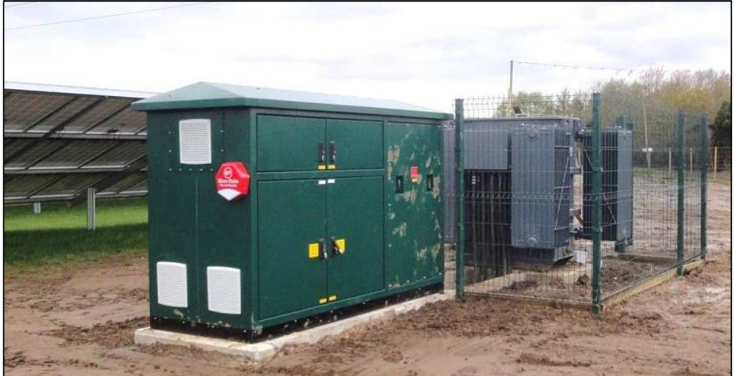
Fig 5: LV switch with transformer
