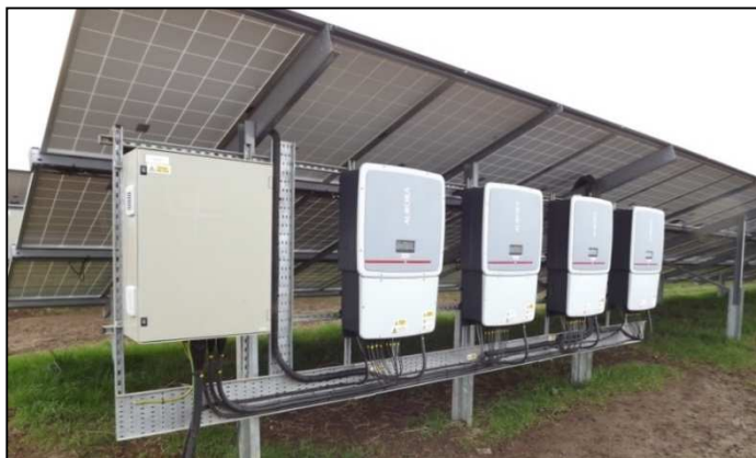
Fig 2: Rear of the array
