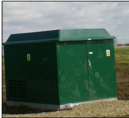
Fig 6: Typical DNO substation
