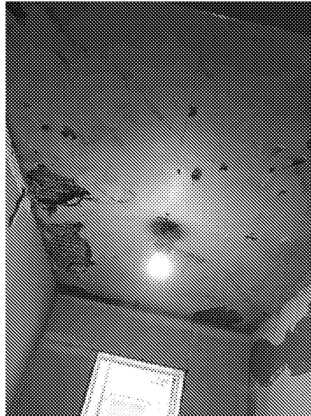
Existing Dilapidated Ceiling
