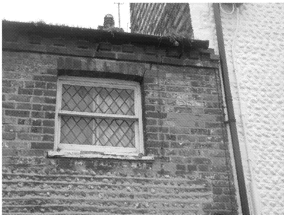
Cracking on brickwork and mortar joints
