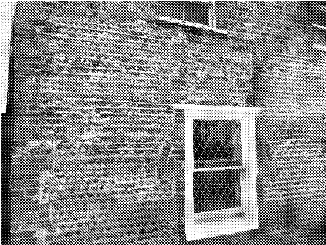
Current condition of pointing.
