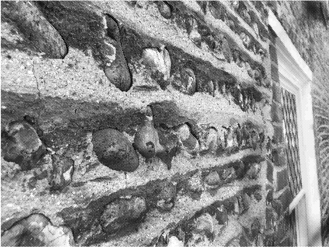
Pointing Coming Away from Wall
