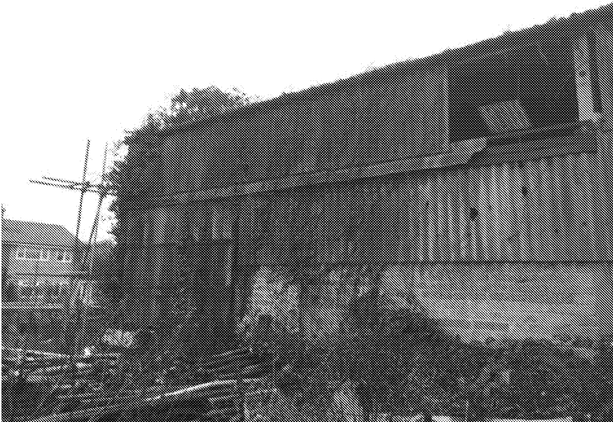
Figure 14. Eastern face of the industrial shed with a broken upper window.
