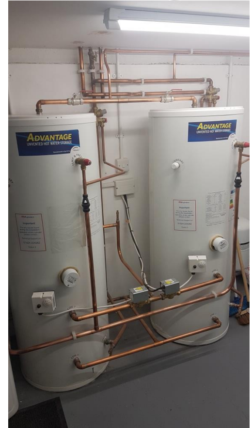
Plant Room 3 - Hot Water Storage Tanks
