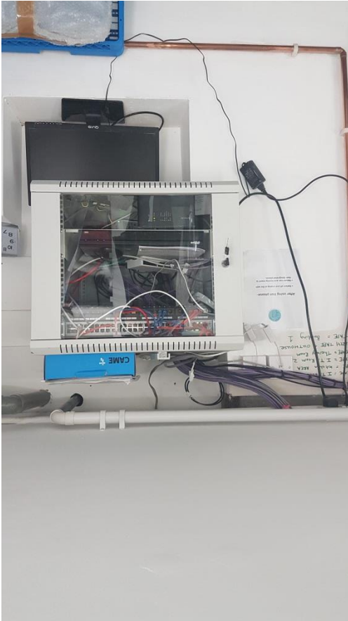
Plant Room 1 - Computer Server
