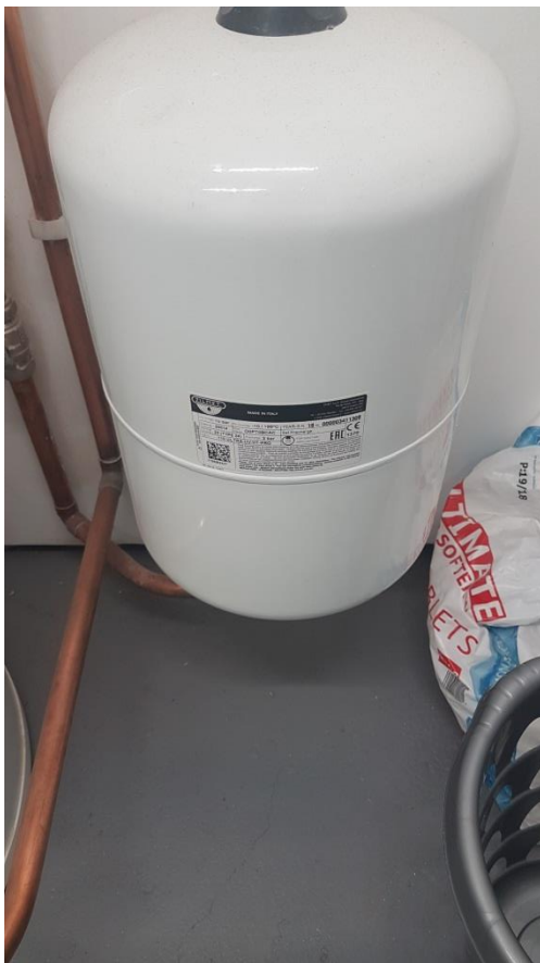
Plant Room 4 – Expansion Pressure Vessel
