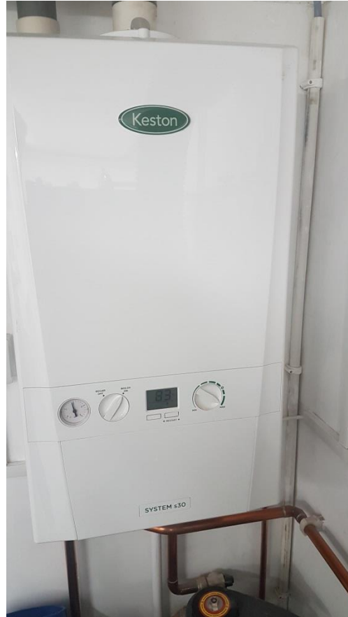
Plant Room 2 – Boiler
