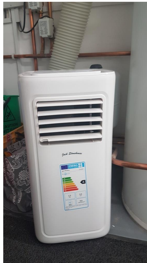
Plant Room 5 – Portable Air Con Unit
