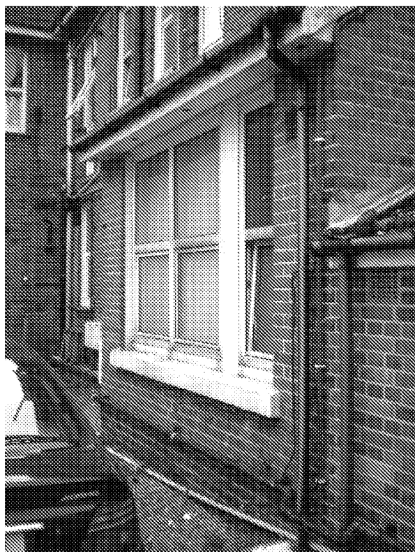
The east (rear) elevation of the west wing. Later (1912 – 1938) extension with wide windows. Aluminium window frames – harmful modern alteration.
