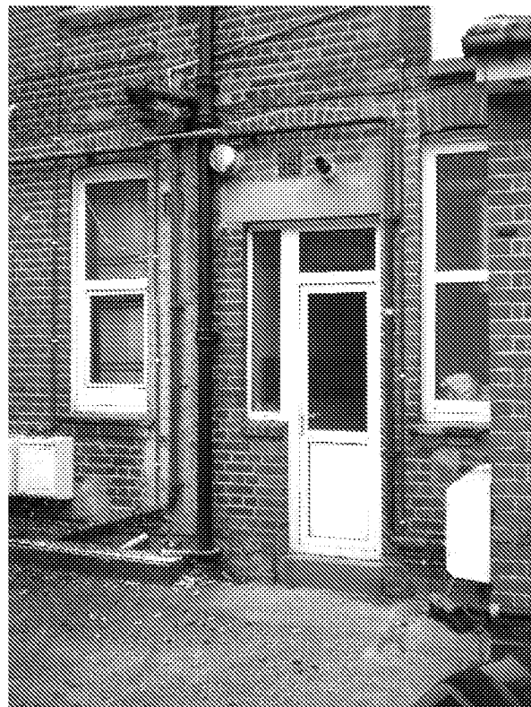
Position and height of door and side window altered and modern window frames – harmful modern alterations.
