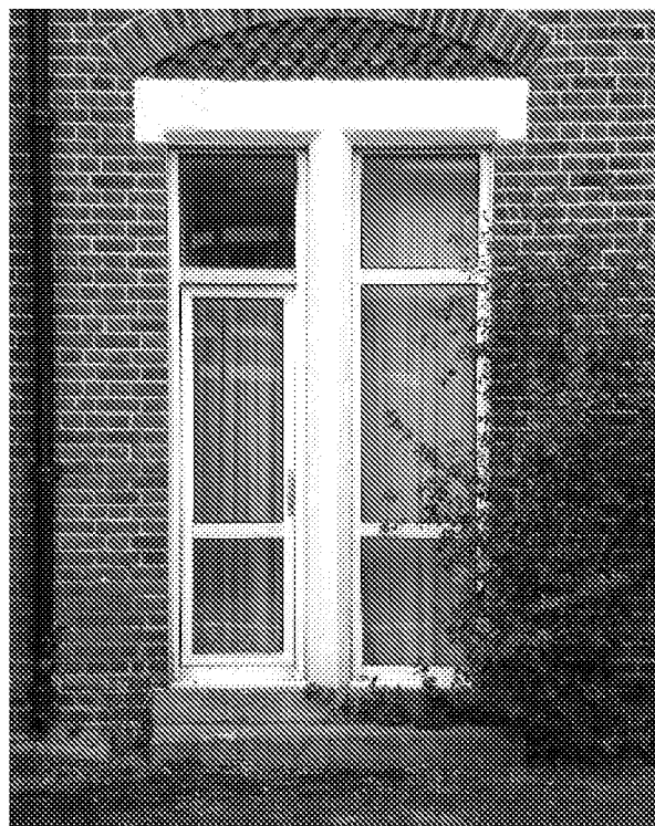
French doors - Modern frames a harmful alteration.
