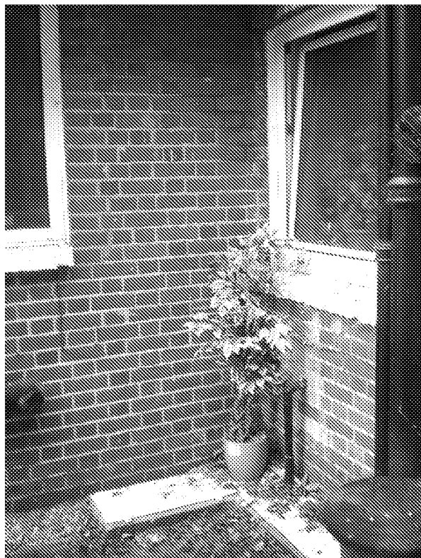
Modern cills and window frames – harmful modern alterations.
