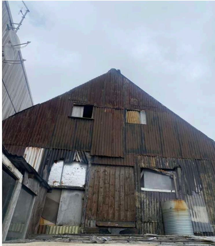
Photograph 10: Close up of the existing garage on Site shown to be in a dilapidated state.
