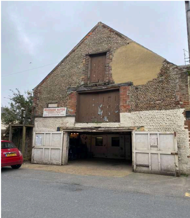
Photograph 1: Derelict garage in the north of the Site as seen from River Road, facing southwest.
