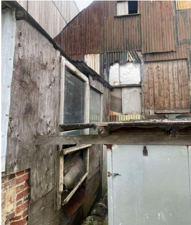
Photograph 9: Close up of the existing garage on Site shown to be in a dilapidated state.
