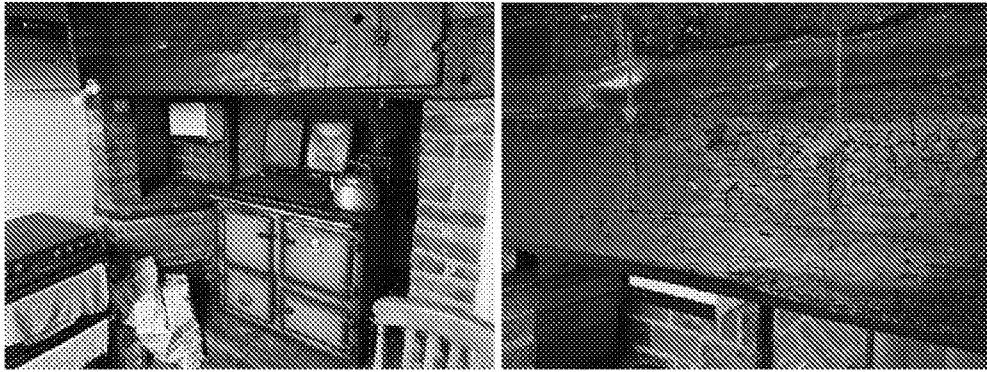
The beam over the AGA with taper burns that predate this part of the building
