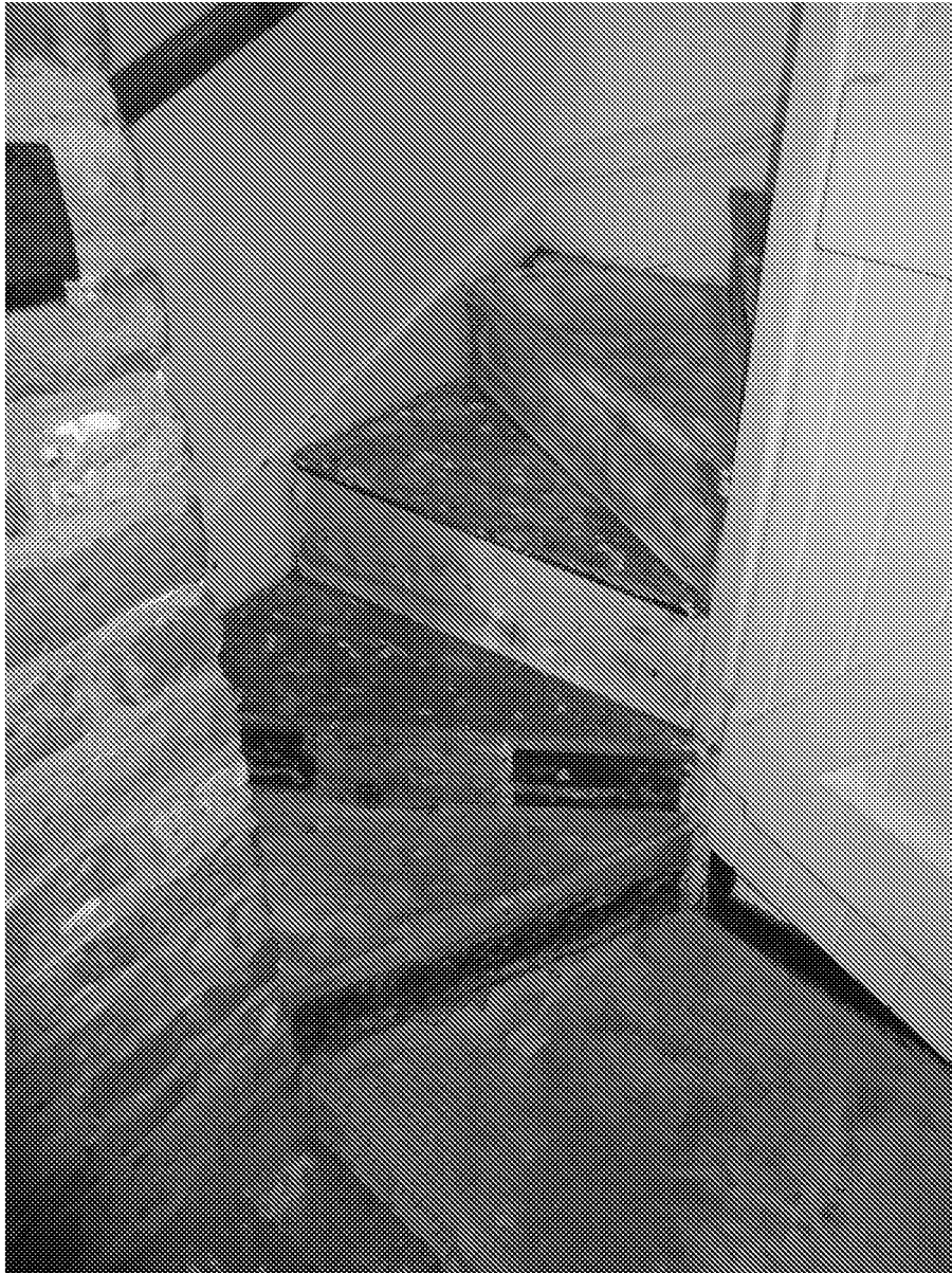
Stairs to be replaced
