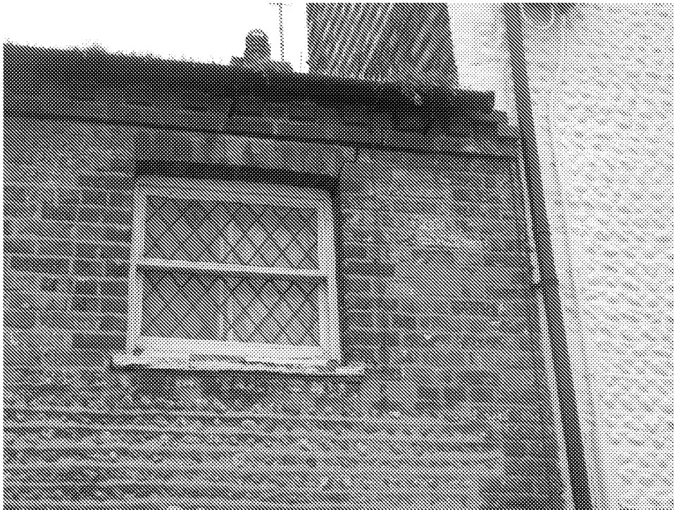
Cracking on brickwork and mortar joints
