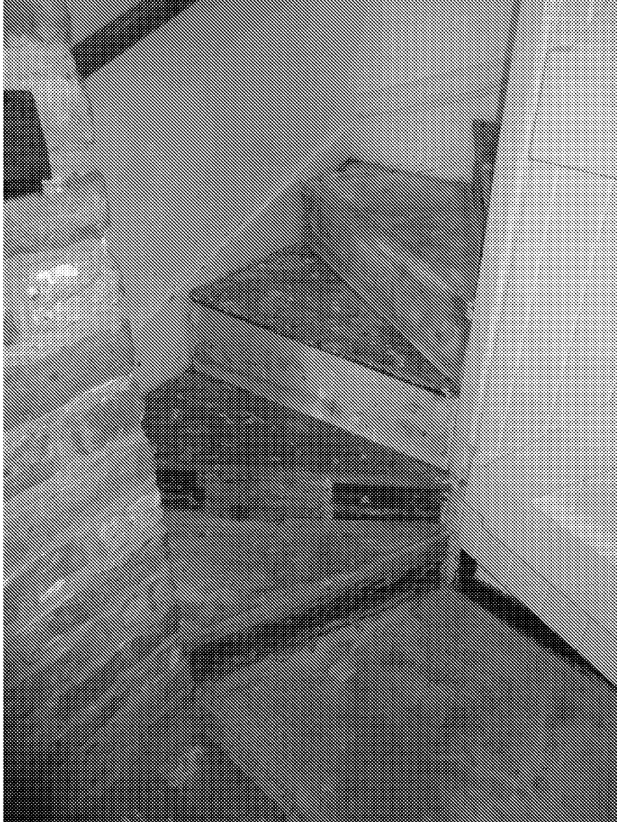
Stairs to be replaced
