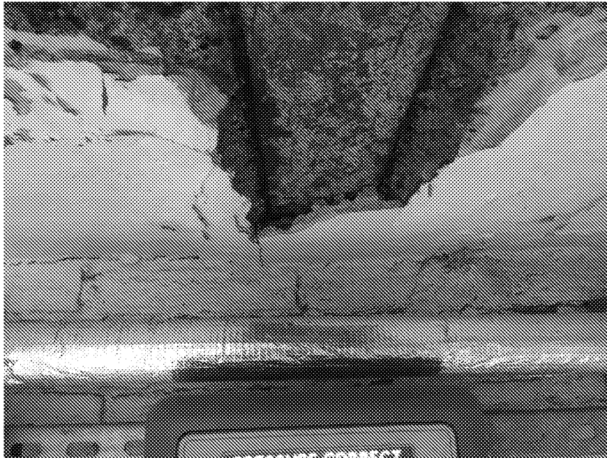
Photo 3 – Corroded Steel Beam
