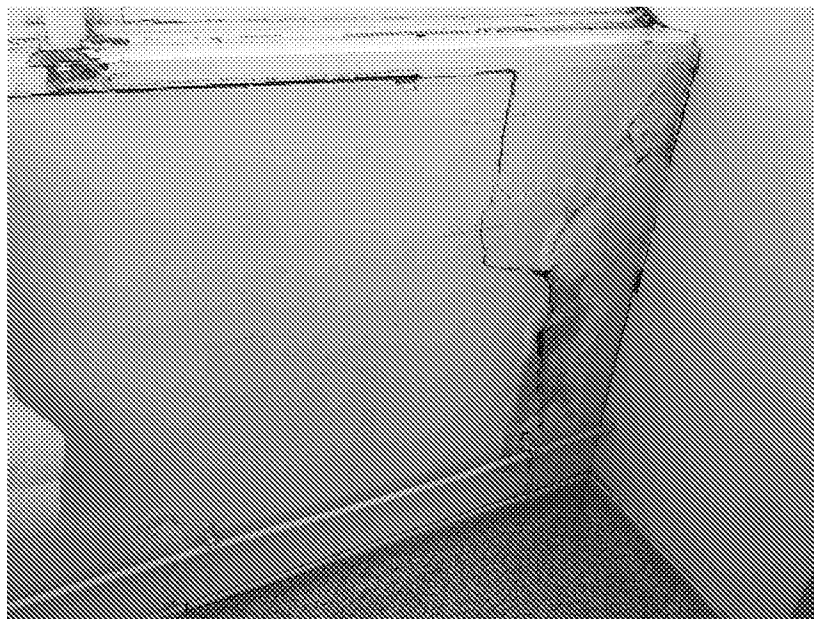
Photo 2 – Cracking within ground floor WCs
