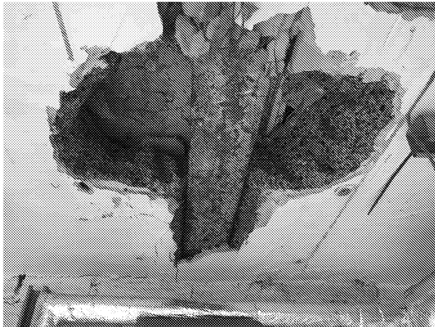
Photo 4 – Corroded Steel Beam
