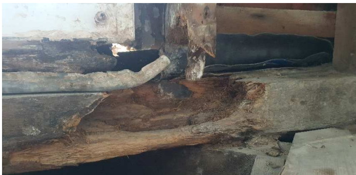
Large gaps in cladding and a poor flashing detail
