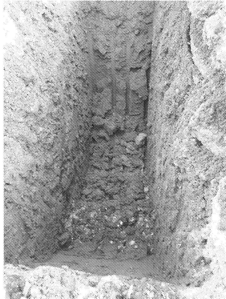
Plate 14: Concrete obstruction in FP1
