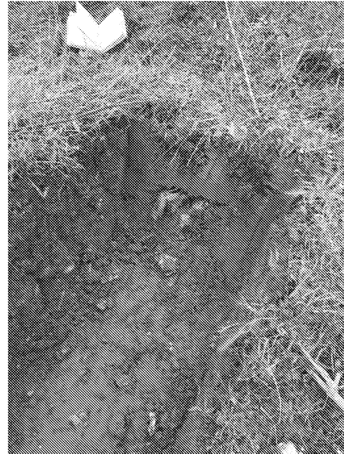
Plate 8: Electrical warning tape in TP207
