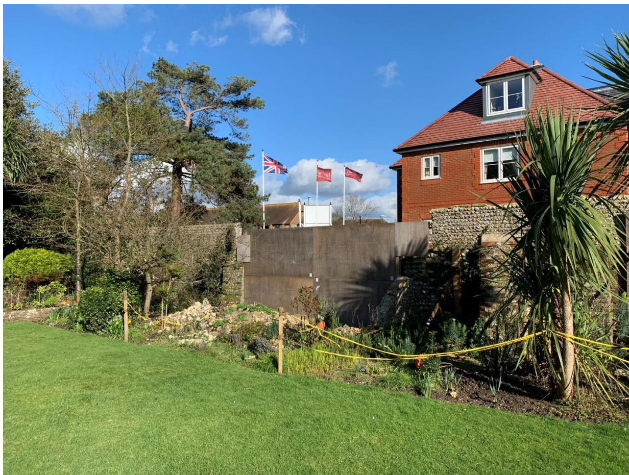
Temporary hoarding between the collapsed section of wall
