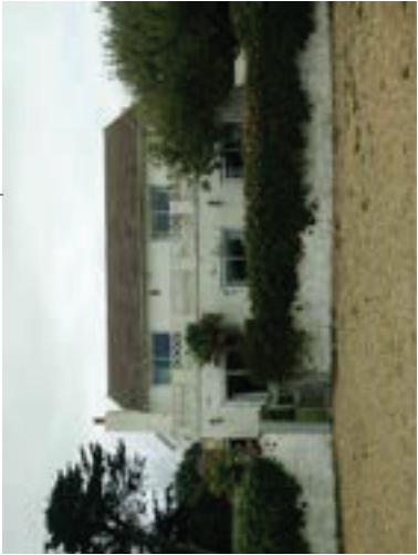
Existing render lattice
