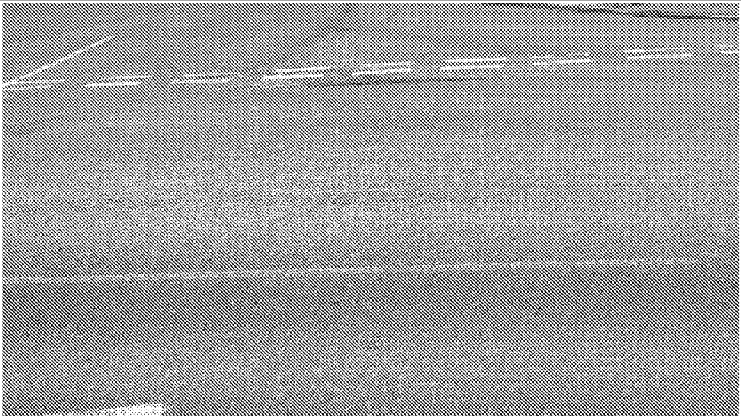
Photo M Ford Road carriageway markings illegible
