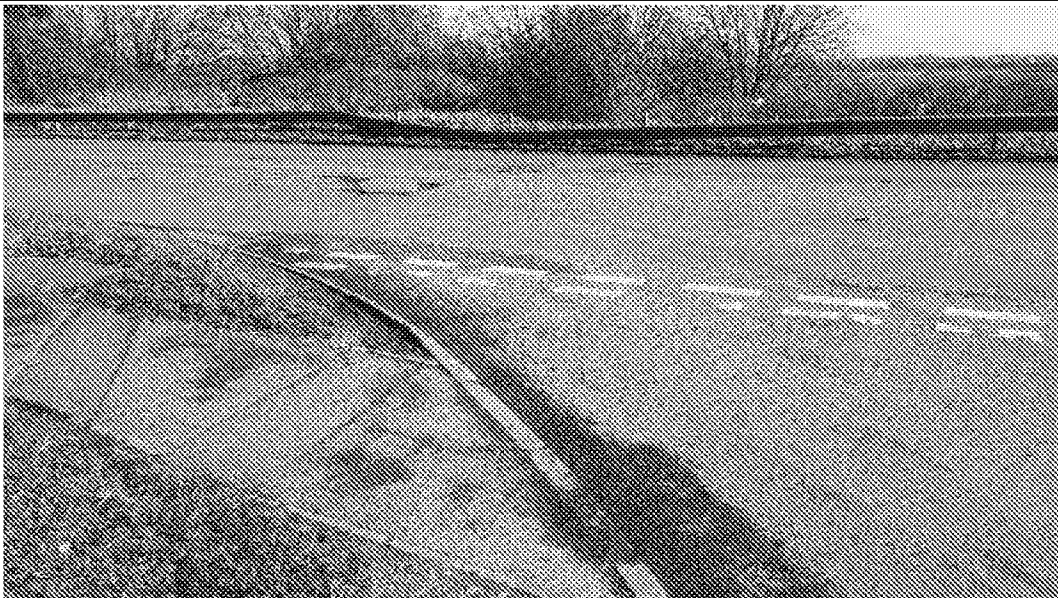
Photo J Ford Road carriageway markings illegible
