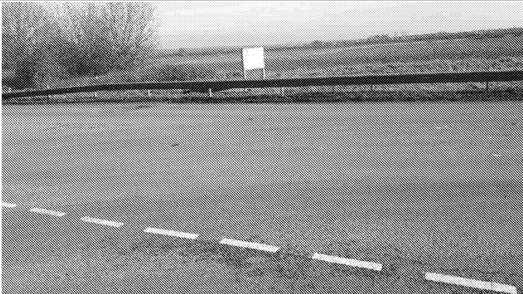
Photo L Ford Road carriageway markings illegible
