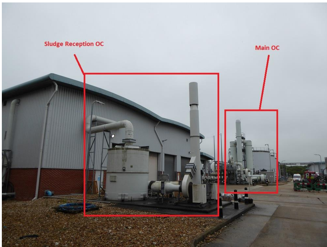
Figure 4-2 Ford WwTW Odour Control.
