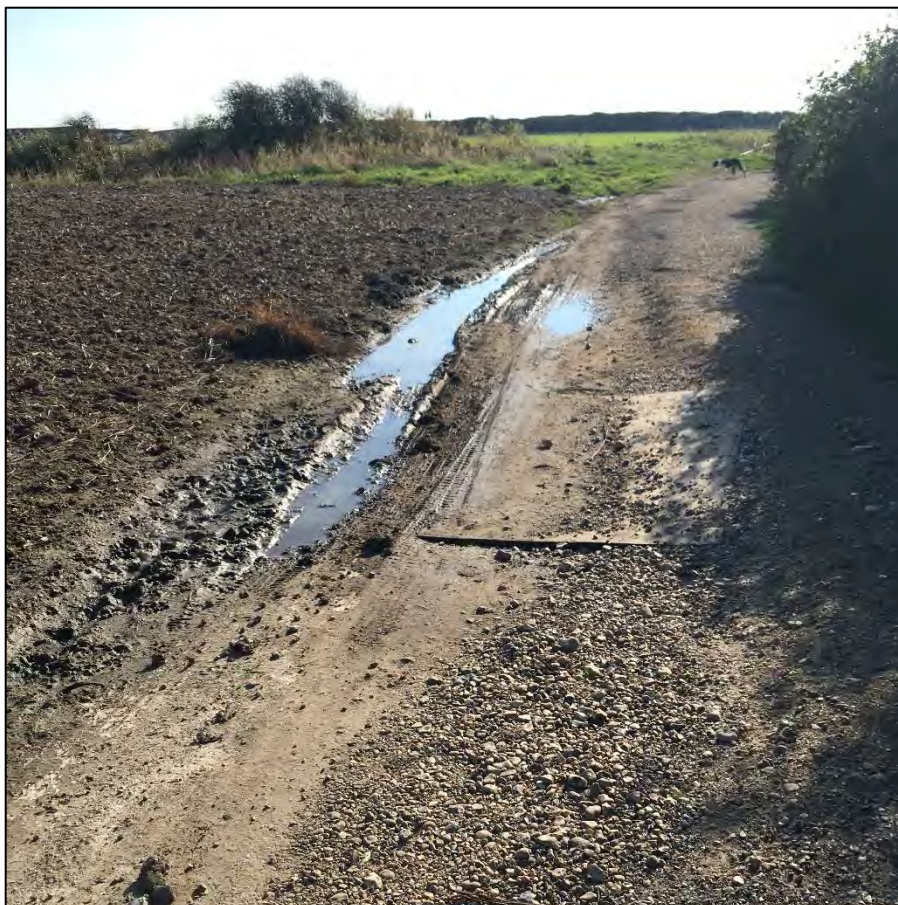
Image 2.12: Uneven Track Surface
