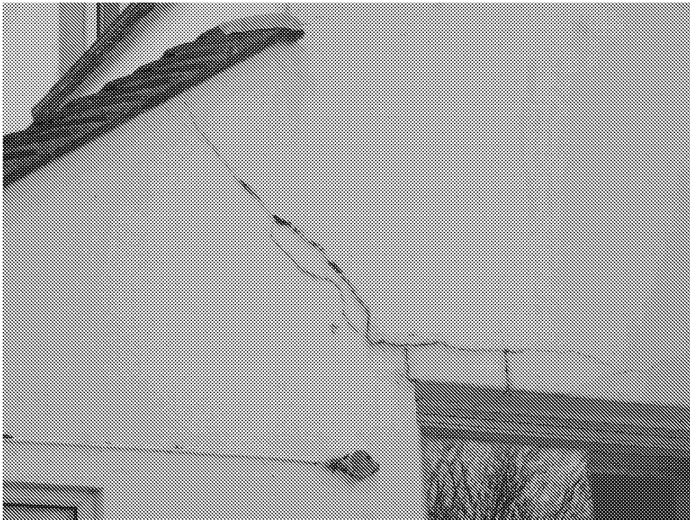
Fig 4 showing cracks in wall at rear of house
