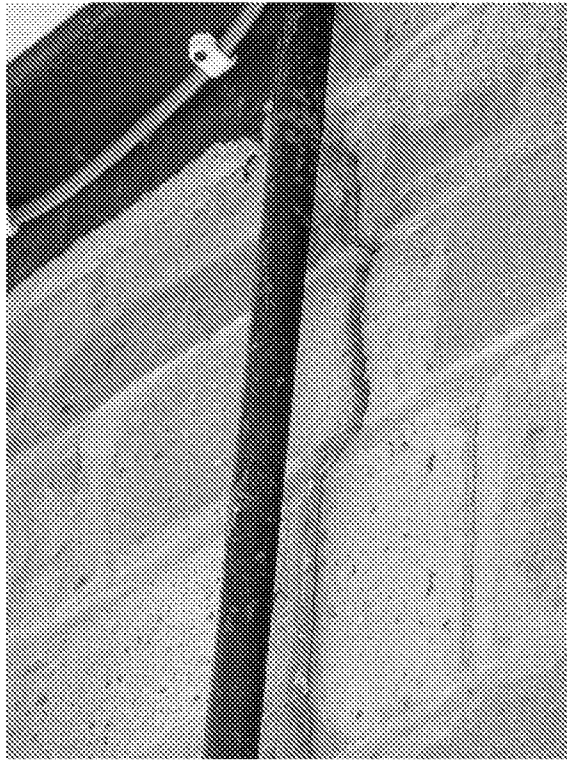
Fig 3 Showing crack in brickwork inside garage.
