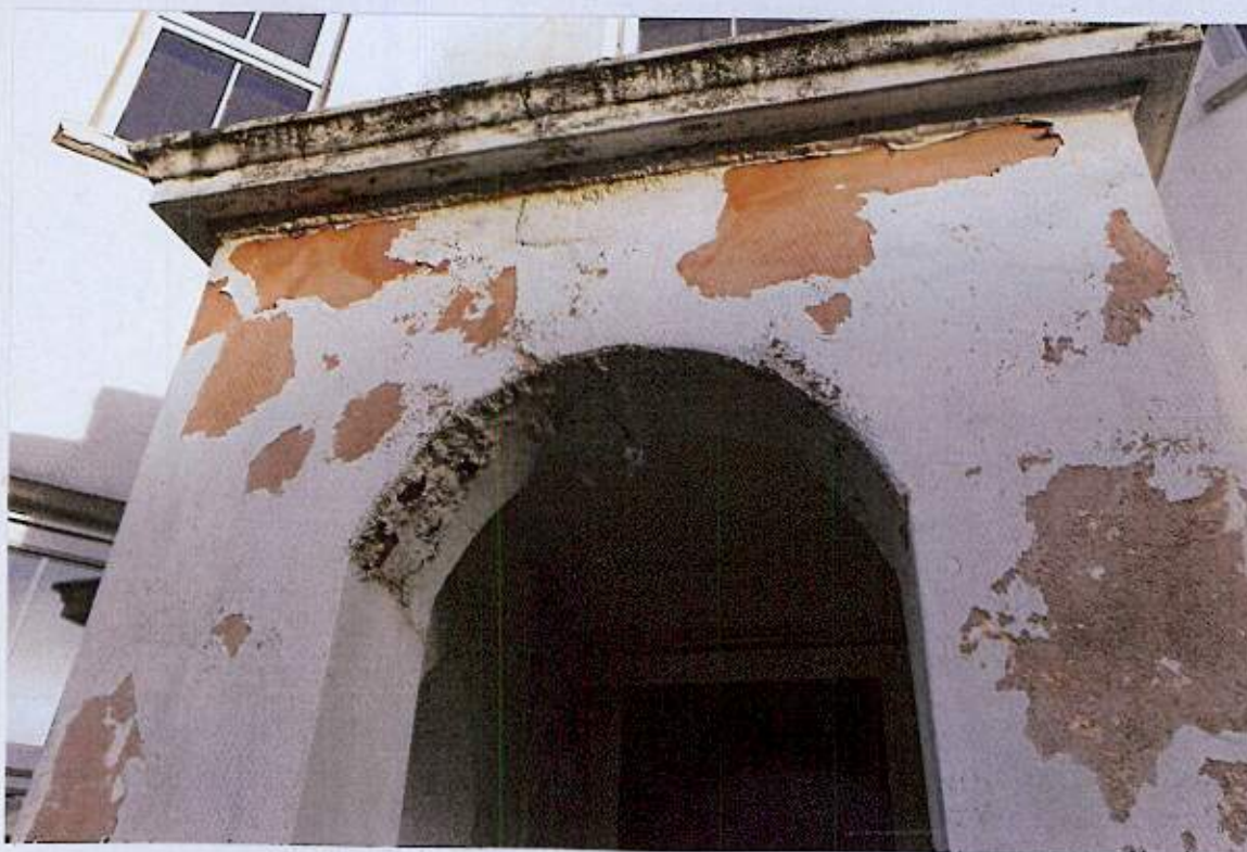
Photo. B – Evidence of fabric deterioration around original front entrance.
