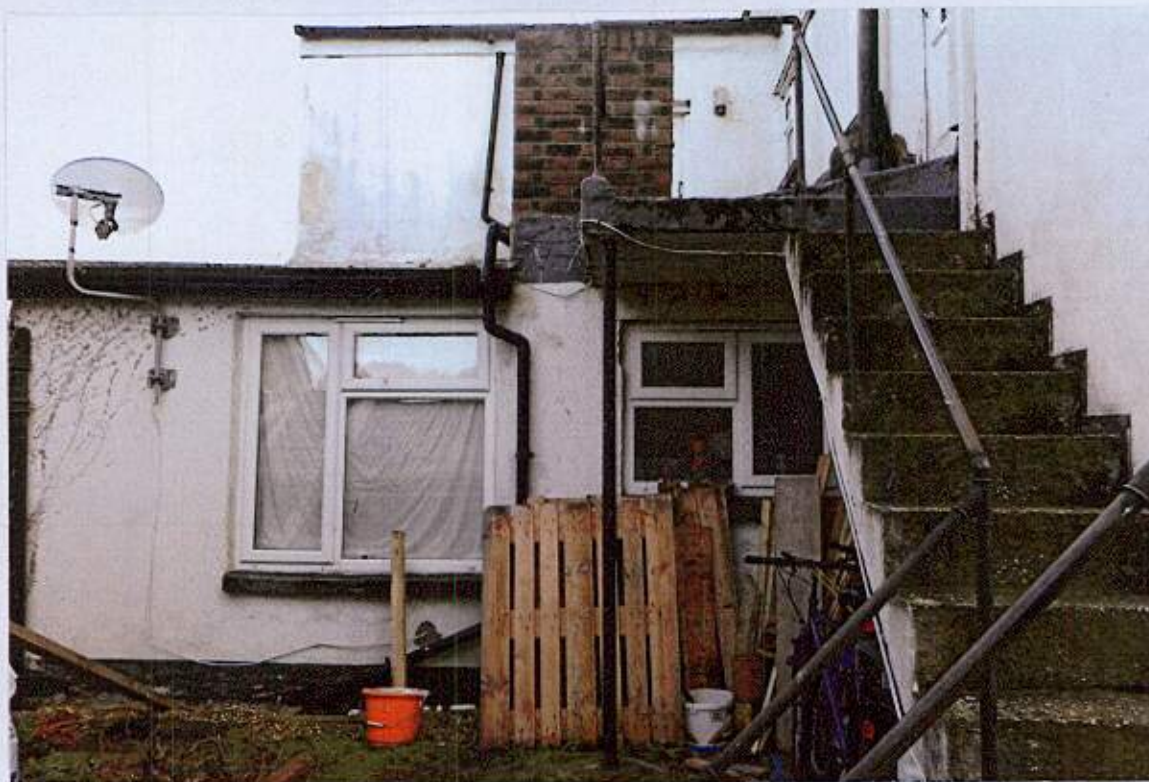
Photo. A- Existing unsatisfactory external concrete staircase to first floor flats.
