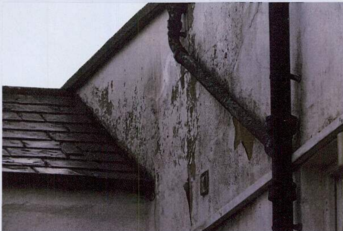
Photo. C - Further signs of external problems around the access to first floor flats.
