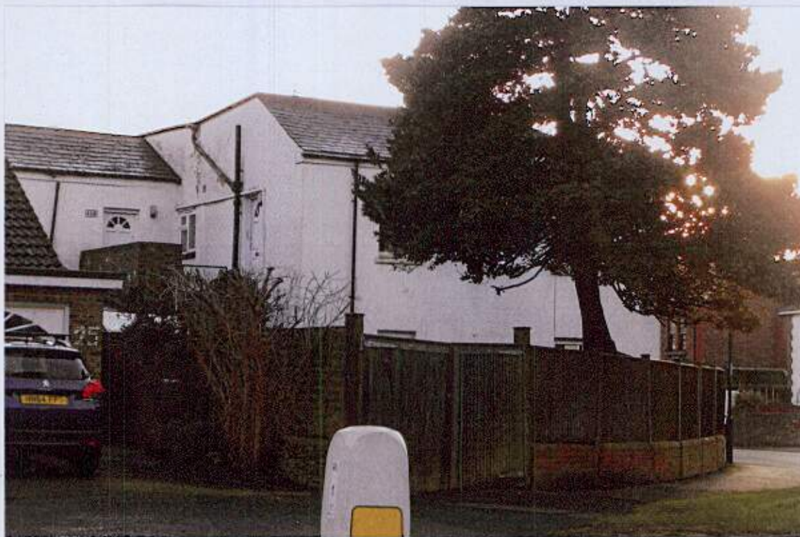
Photo. D - Awkward shaped roof, covering original double pitch, now in poor state.
