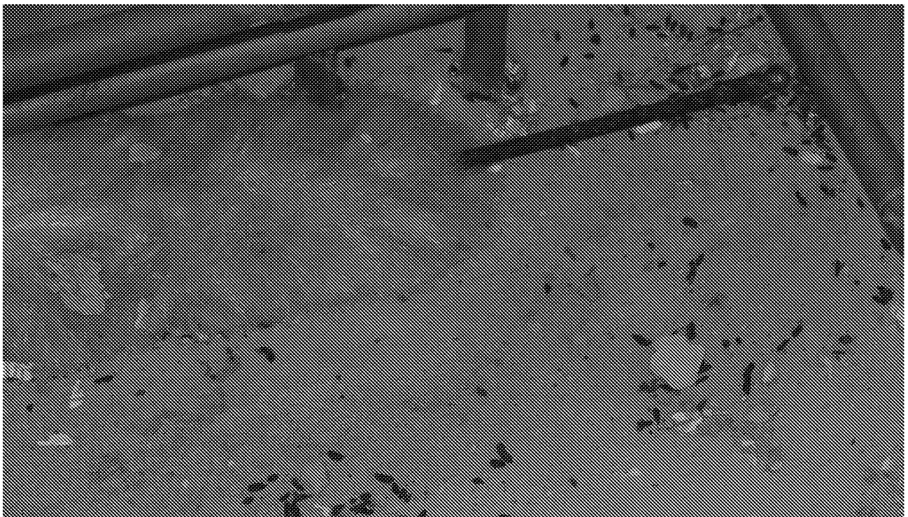
Photograph No. 10 - There were a number of rat droppings within voids in the Building B1 but no evidence of bats.
