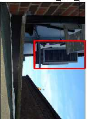
Photo 5 AC as installed
