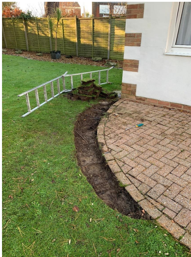
Figures 1 & 2 - Excavation revealing root material to be pruned out to facilitate repair of damaged patio. Photo taken: 08-Dec-2020.
