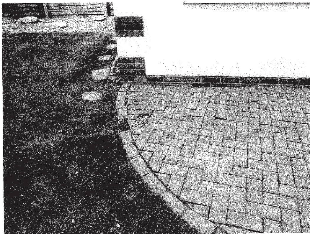
Patio in July 2020 with increased unevenness
