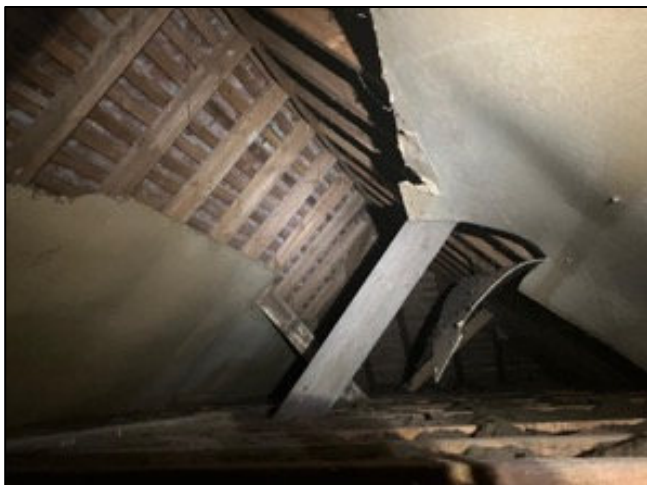
Photograph 30 Peeling boards in Void 4
