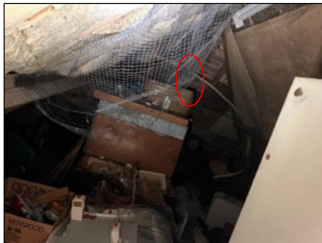
Photograph 25 Void 3 in the main house, note the exposed roof tiles
