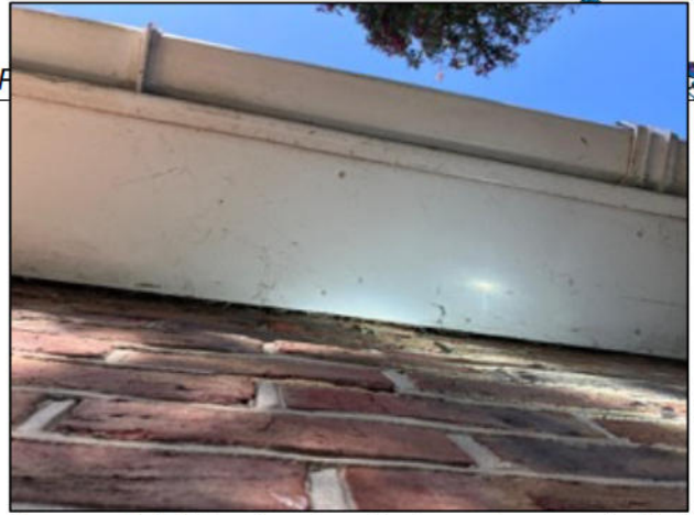
Photograph 13 Heavily cobwebbed gap between the brick work and soffit box on the southern elevation of the house
