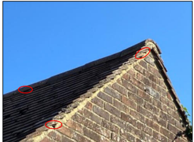
Photograph 17 Gaps in the mortar on the house's western elevation
