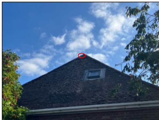
Photograph 21 gap beneath a ridge tile on the northern elevation
