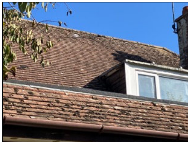
Photograph 19 hanging tiles on the west-facing dormer window and missing/lifted tiles on the west-facing roof pitch. Note the guttering blocking access to any gaps along the edge of the ground-floor roof.
