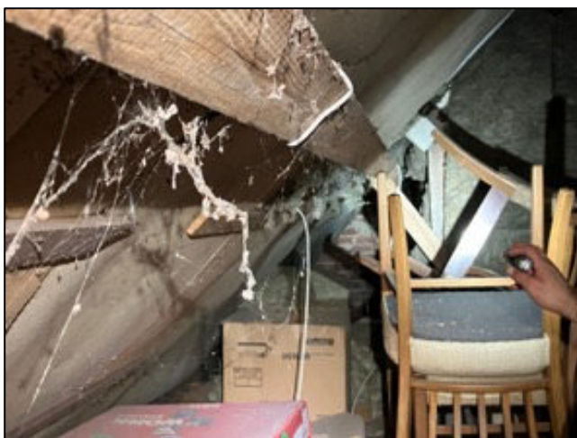
Photograph 26 Cobwebs in Void 3
