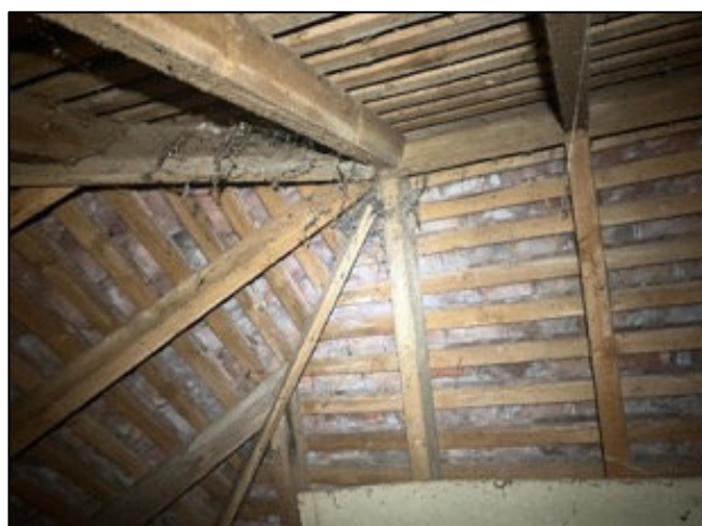
Photograph 29 Exposed tiles and cobwebs in Void 4
