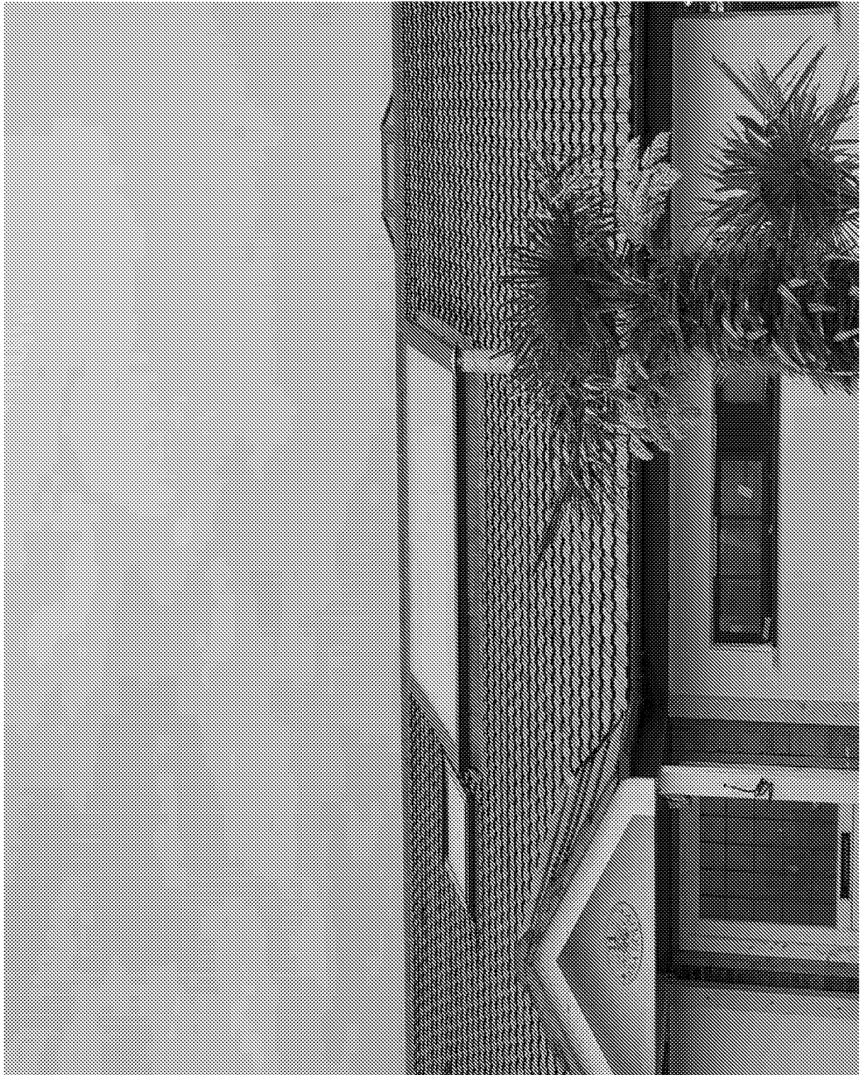
Fig 10 - Large rooflight which is not in the plans permission was granted for
