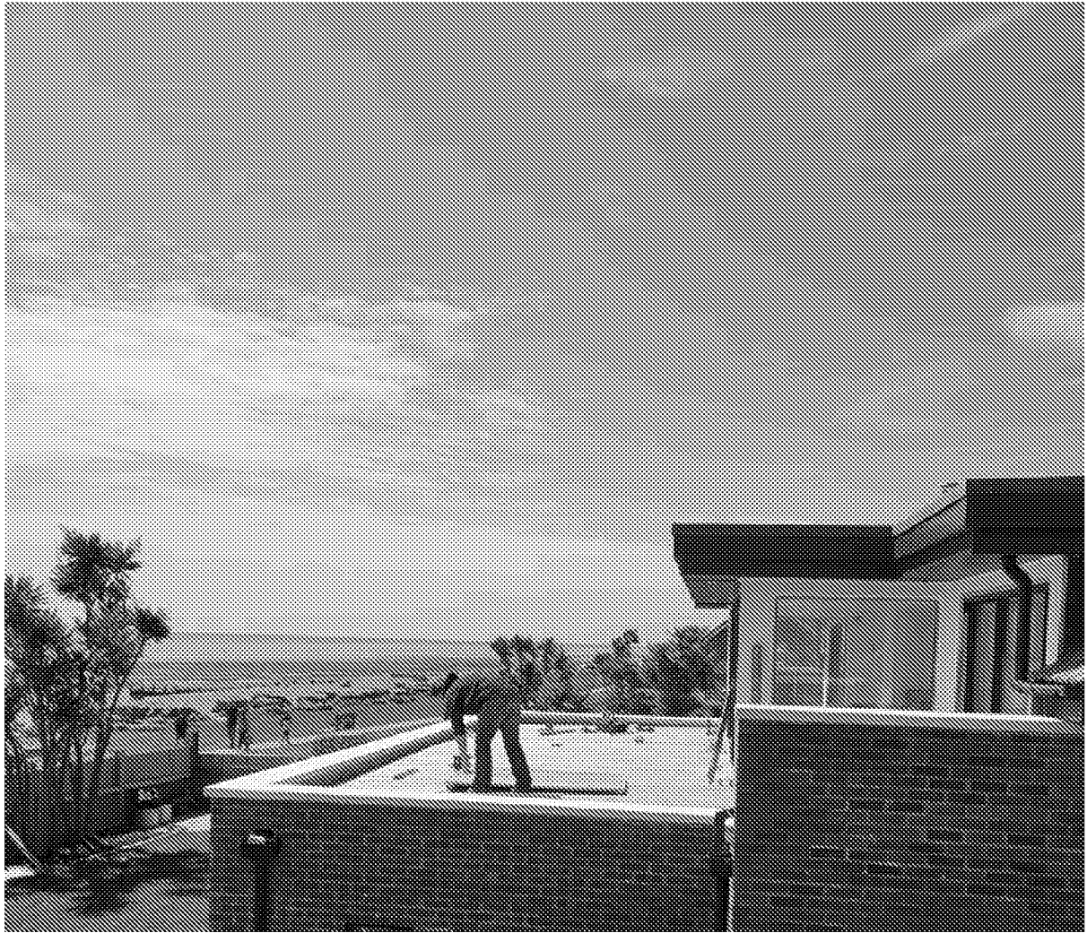
Fig 8 - Wooden decking completed on entire ground floor roof, against requirement for green roof and covering entire roof which even now permission is not being sought for
