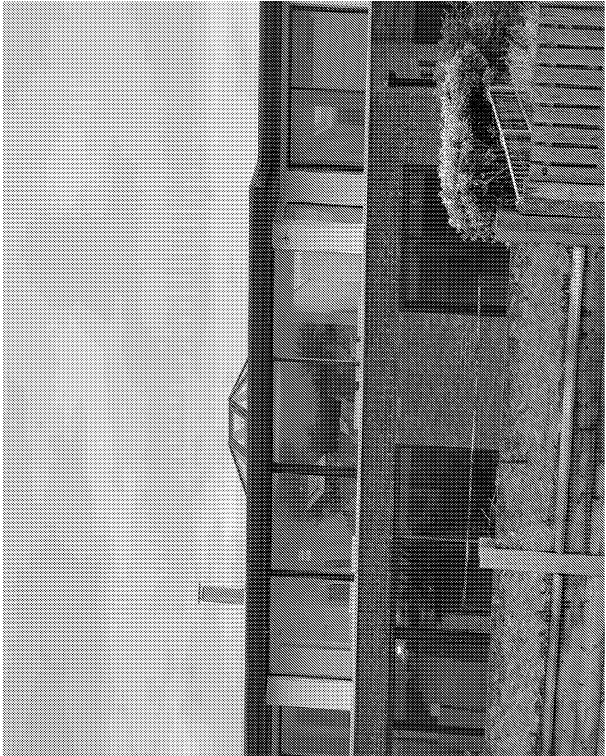
Fig 11 - Large porch extending past current building line towards road, not in plans permission granted for
