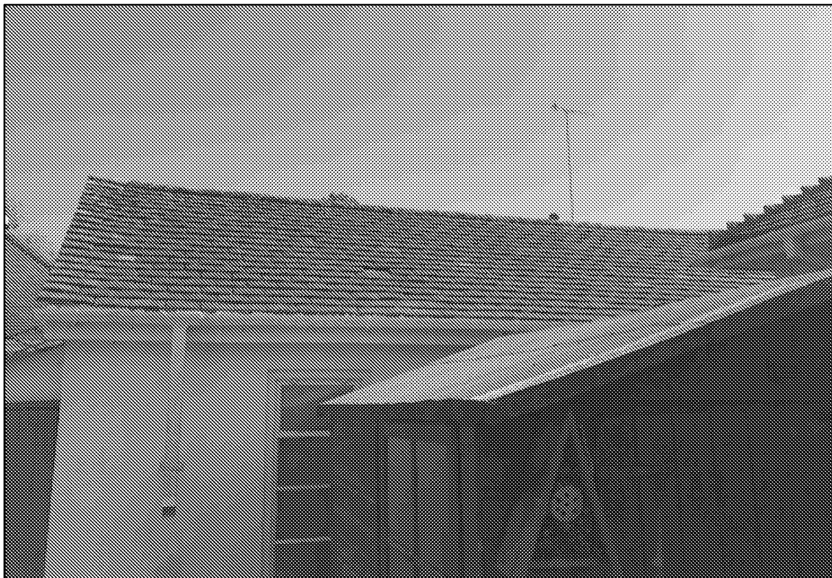
Photograph 5. The northern elevation of the small garage, with a single cracked tile visible.
