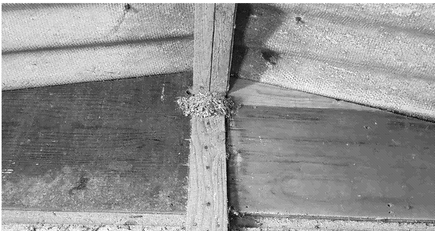
Photograph No. 8 - Swallow nest located to the northern section of Building B4.
