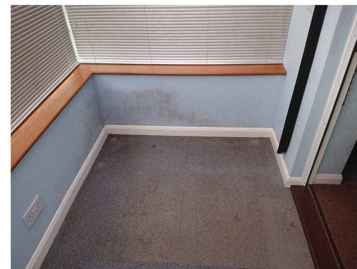
Existing porch (penetrating damp)
