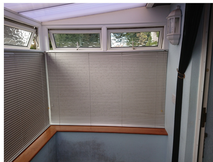
Existing porch (penetrating damp)
