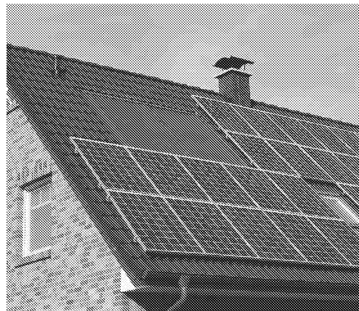
Making best use of South orientation by use of photovoltaic panels
