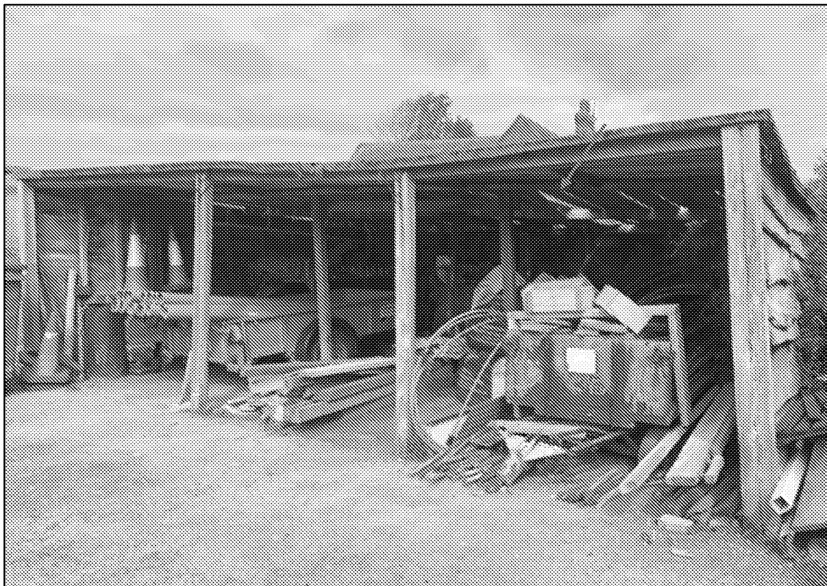
Photograph 5. Showing Building 4. Note the poor condition of the timber sarking and bitumen lining on the roof (red arrow).
