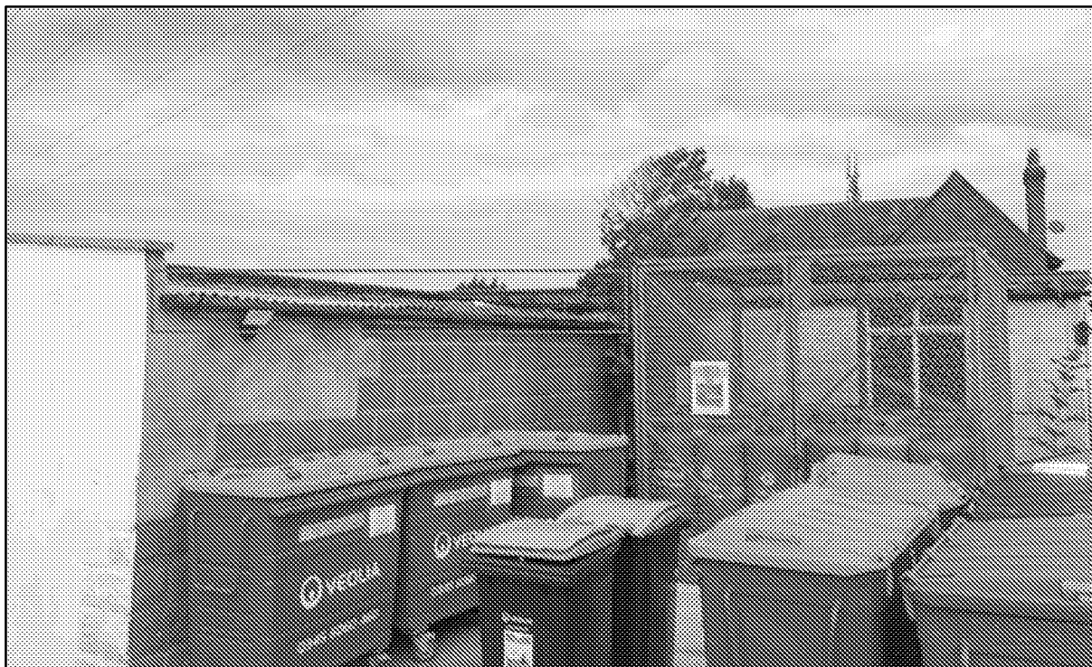
Photograph 2. External view of Building 2 (part obscured behind the metal cage). Note the flat roof with mixed corrugated chrysotile and metal roofing sheet with gaps where sheets overlap (red box).
