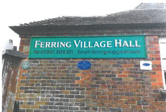
CURRENT MAIN SIGN TO BE REPLACED WITH NEW
