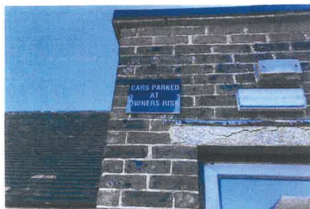
TO BE REPLACED WITH 1 GENERAL PARKING SIGN
