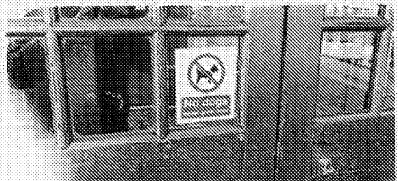
TO BE REPLACED WITH NEW
