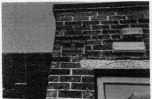
TO BE REPLACED WITH 1 GENERAL PARKING SIGN
