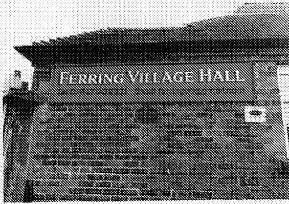
CURRENT MAIN SIGN TO BE REPLACED WITH NEW
