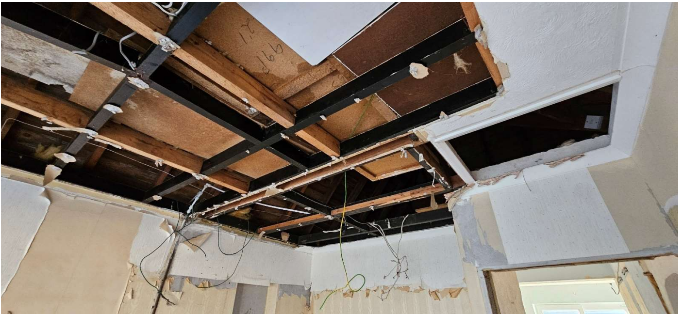
Photo 7 – Removed plasterboard in front room allowing for access between the living space and loft void
