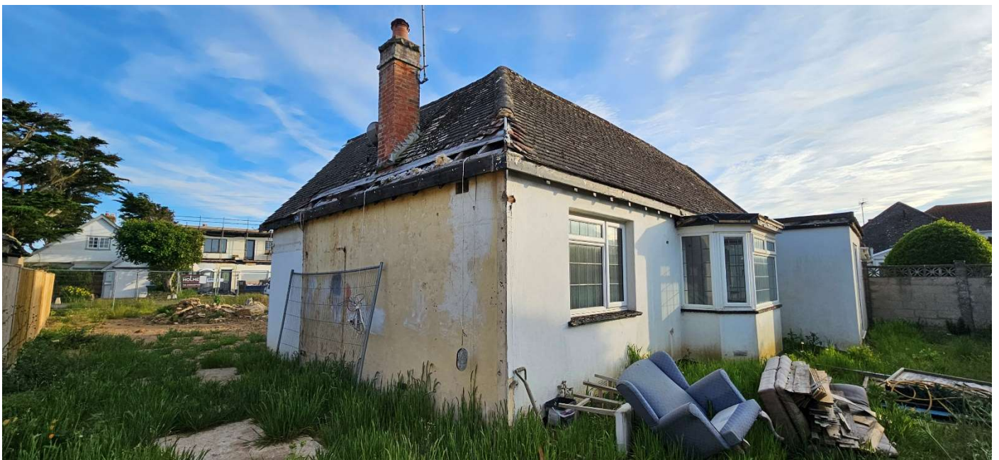
Photo 2 – Northeast corner of the building with significant volume of missing roof tiles
