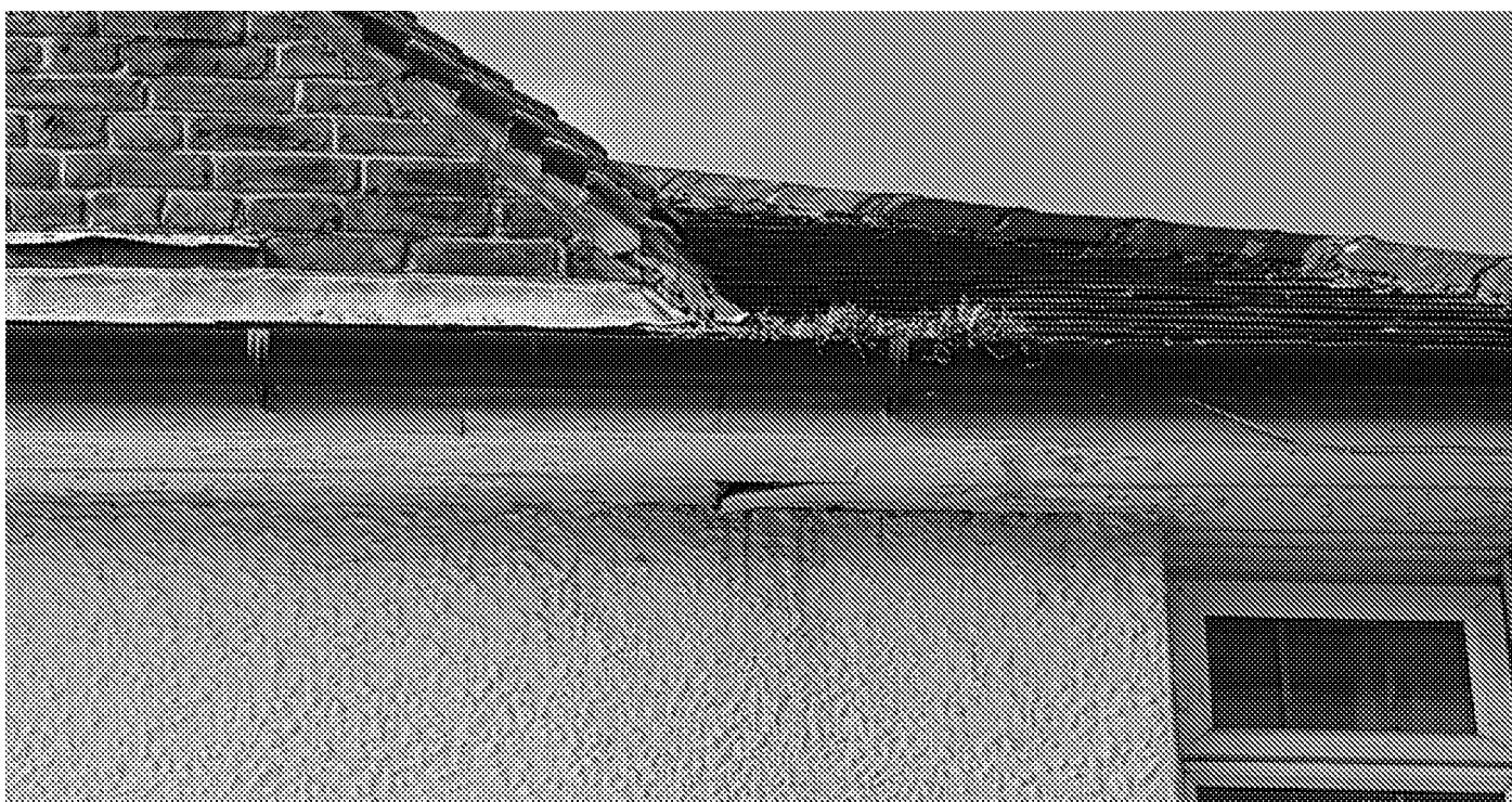
Photograph No. 6 - Small gap at soffit which could possibly allow some bat access.
